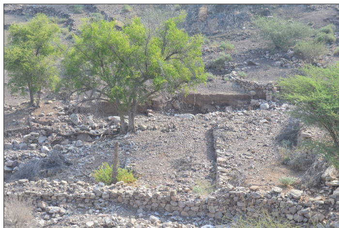
Figure 3. Eroded agricultural terraces and collapsed terrace walls at Suhaila 3
